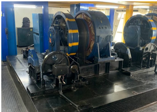
Fig. 15. Elevators with high energy-consuming electric motors
