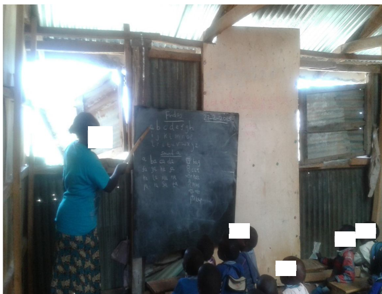
Figure 6 A pitiable structure of one classroom
