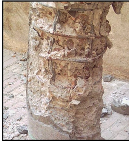
Fig. 14 Failure of helices
